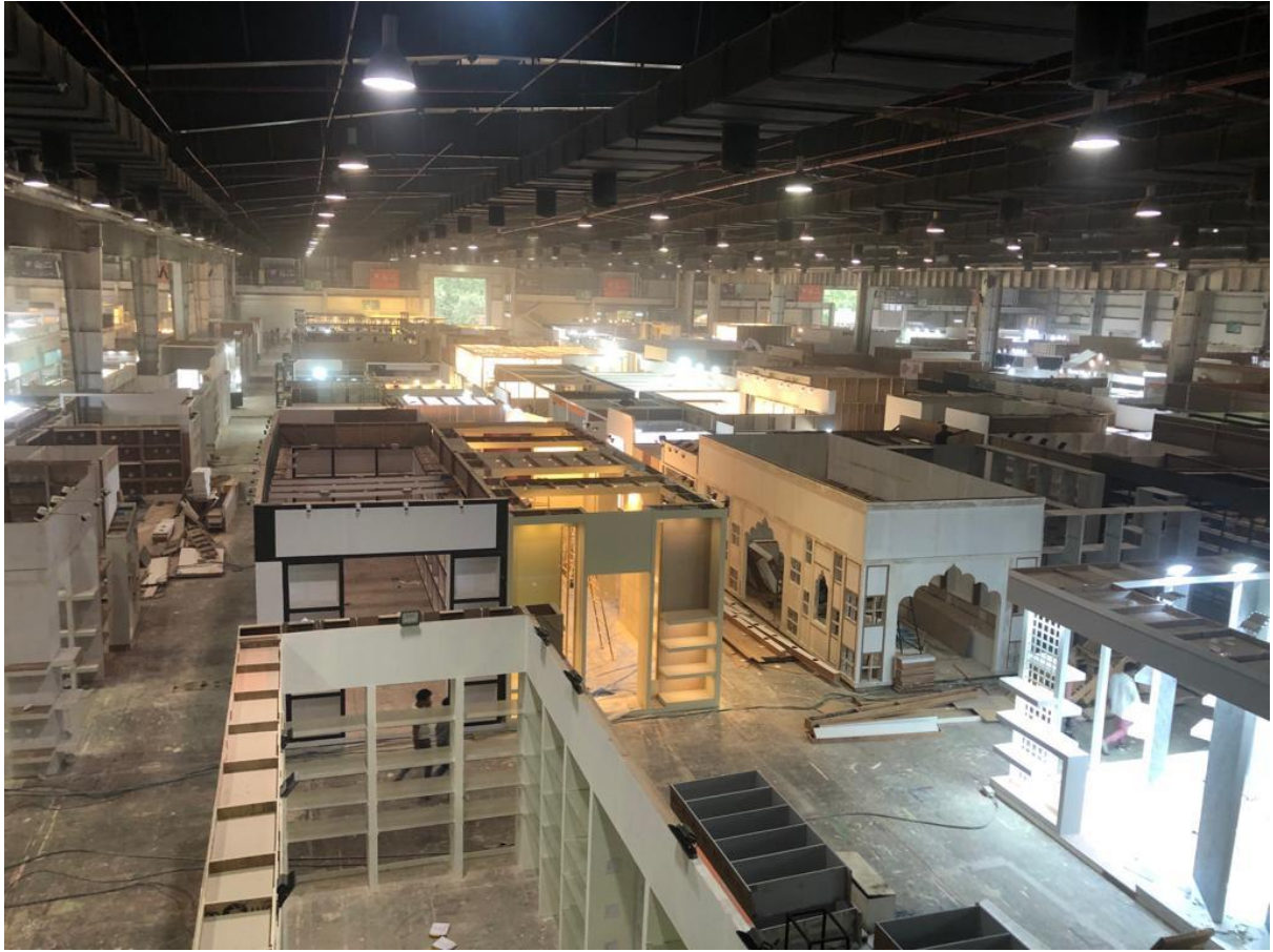
PHOTO - 4 - 54th IHGF Delhi Fair Autumn'22 construction is in full swing at India Expo Mart, Greater Noida to be organized from 14-18 October'22
